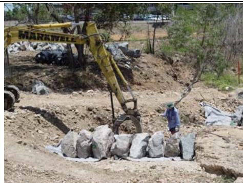
Solander Road rock ramp cascade fishway – placement of ridge rock on prepared foundation (08/12/05)
