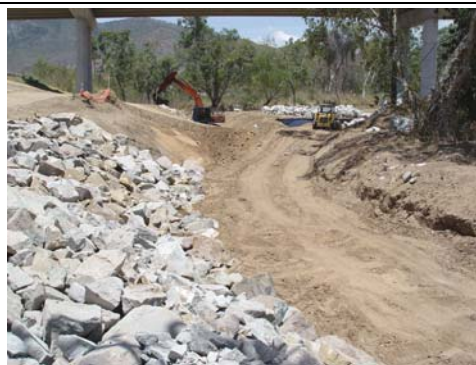
Douglas Arterial Project – trapezoidal diversion drain before construction of rock ramp fishways for grade control (21/10/04)
