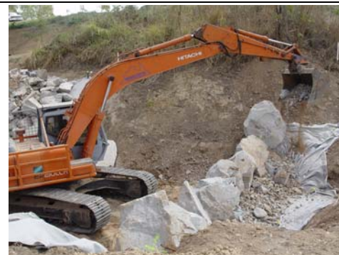
Douglas Arterial Project rock ramp fishway – placement of gravel fill to stabilize ridge rock and as foundation to apron rock (21/10/04)
