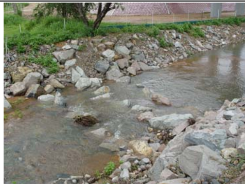
Douglas Arterial Project rock ramp fishway within open channel diversion drain at bridge site (25/01/05)
