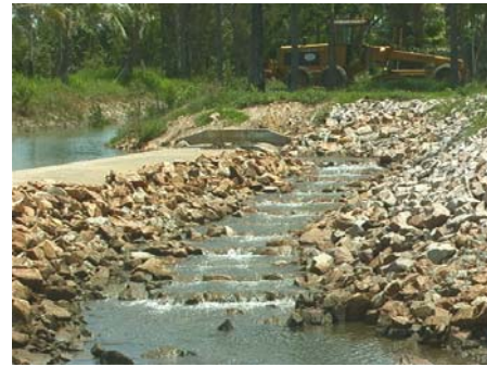
Port Hinchinbrook, Cardwell rock ramp fishway at weir – ridge rock design (Source: Tim Marsden)
