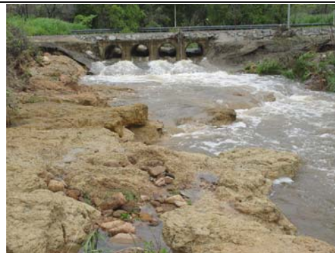
Solander Road culvert / causeway – fish migration barrier problems in channel downstream of crossing (15/01/04)
