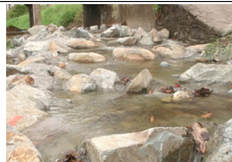
Reliance Creek, Mackay rock ramp fishway at road culvert – showing grouted rock channel (Source: Marsden et al. 2003)
