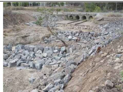
Solander Road rock ramp cascade fishway – looking upstream to rock ridge / cascades # 1 and #2 after construction (17/12/05)
