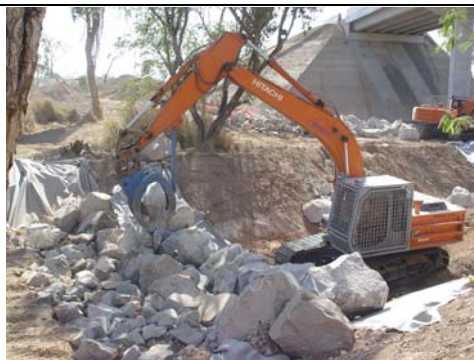
Douglas Arterial Project rock ramp fishway – looking downstream during construction of rock ridge and apron (21/10/04)
