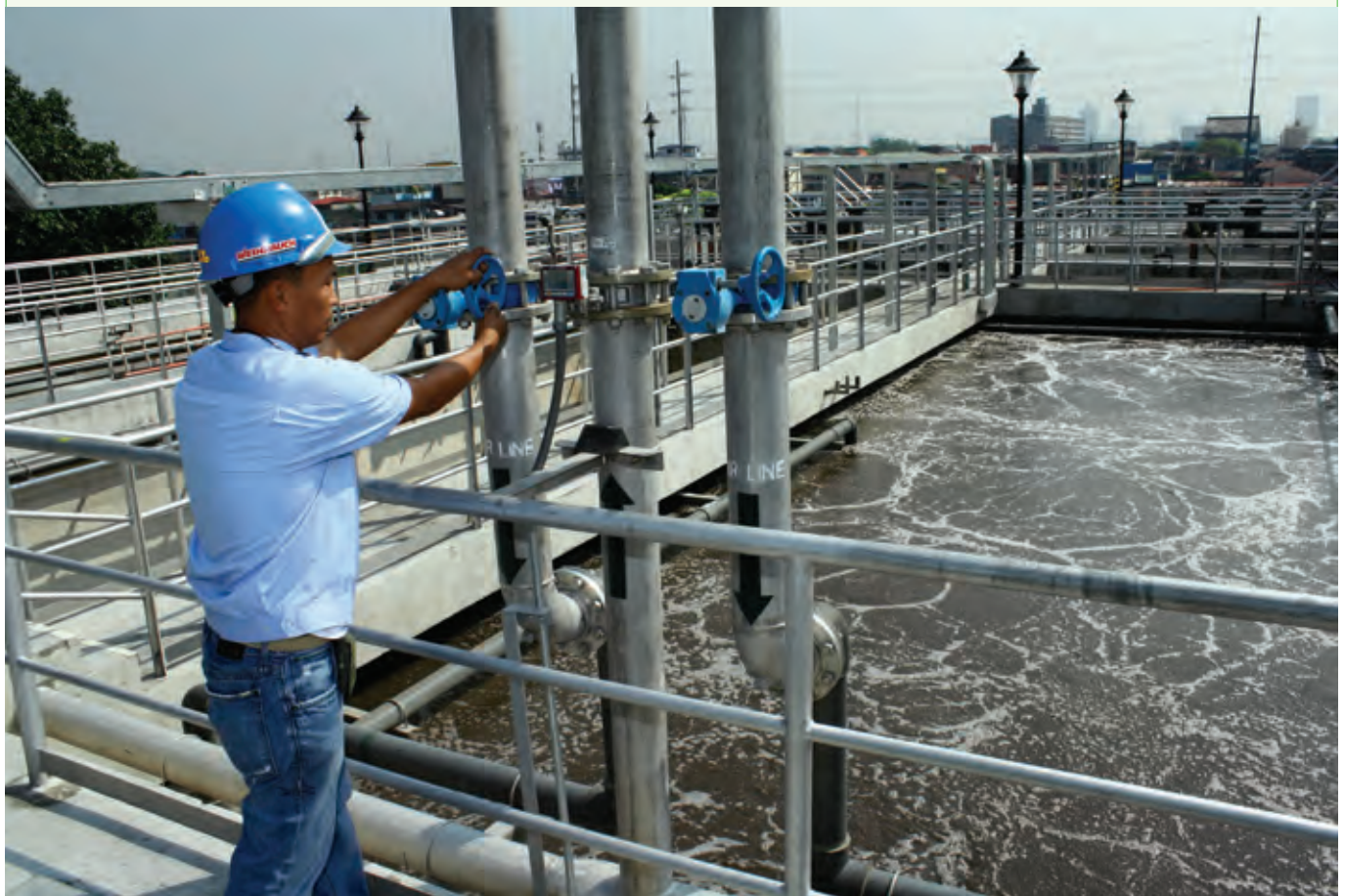
Water treatment plant, Philippines. Image: Danilo Pinzon, World Bank.
