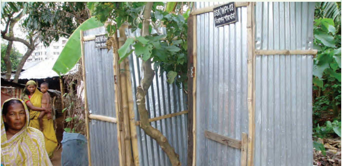
New latrines in Bangladesh. Image: Water.org.
