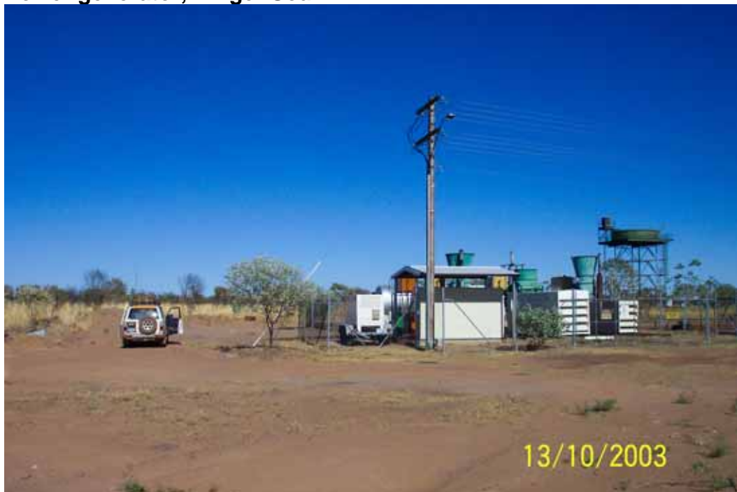
Figure 4.5 Power generator, Ringer Soak
