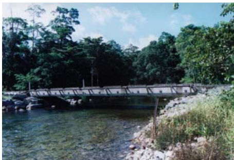
Bridge developed as remediation of previous culvert crossing in north Queensland stream (Source: Ross Kapitzke)
