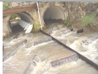
Apron baffle fishway on culvert apron, and corner "Quad" baffle and offset baffle fishways in pipe barrels (09/04/06)
