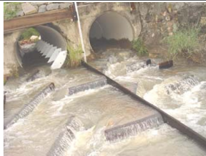
Pipe culvert and apron baffle fishways on Solander Road crossing of University Creek (09/04/06)
