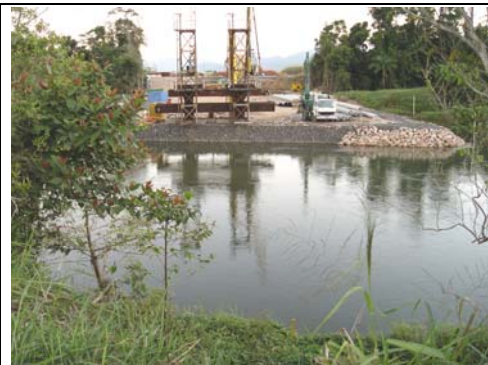
Temporary bund installed with major waterway opening retained during construction of new bridge crossing of the Tully River for Bruce Highway Corduroy Creek project (21/08/07)
