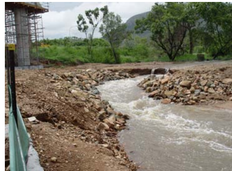
Turbulent high velocity flow downstream of pipe – looking upstream (15/01/04)
