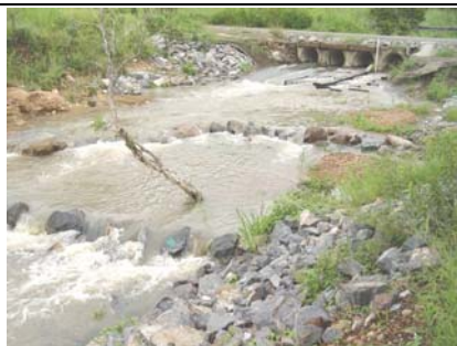
Rock ramp / cascade fishway to overcome water surface drop at culvert apron downstream of culvert (09/04/06)
