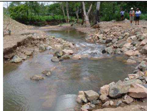
High velocity barriers to fish and erosion at outlet of small diameter bypass pipe culvert beneath temporary road crossing for Douglas Arterial Road crossing of University Creek (17/01/04)
