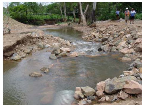
Erosion and turbulent high velocity flow at outlet – looking downstream (17/01/04)
