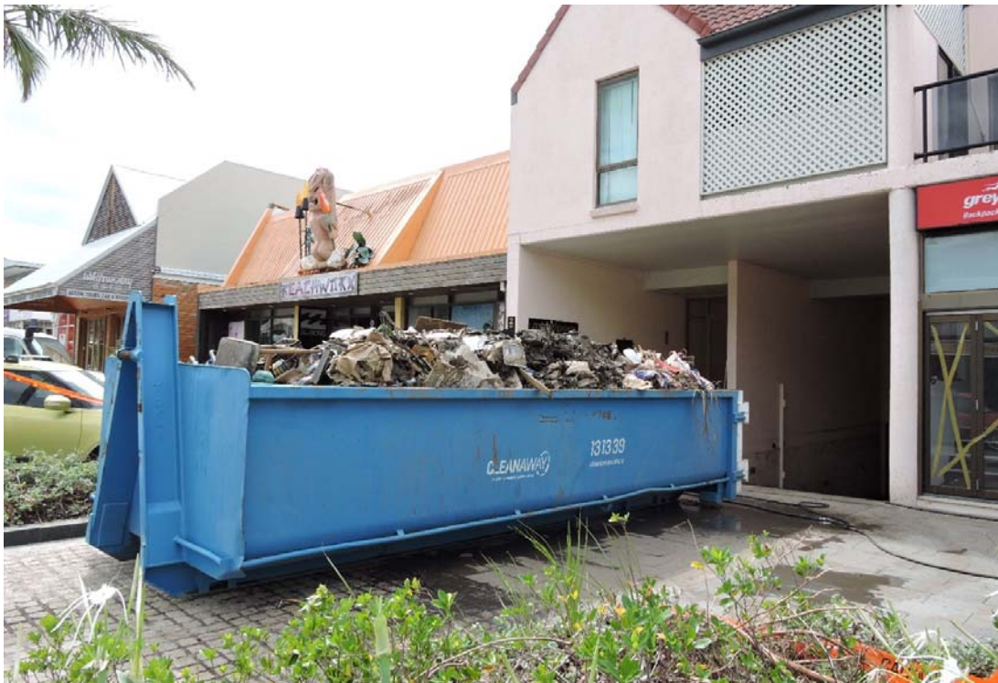
Figure 9. Business clean up post-cyclone and flooding Airlie Beach
