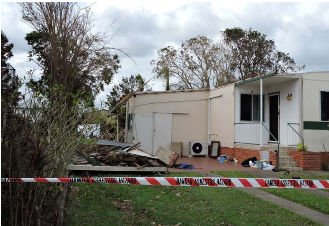
Figure 13. Asbestos identified as a further hazard in damaged housing, Proserpine
