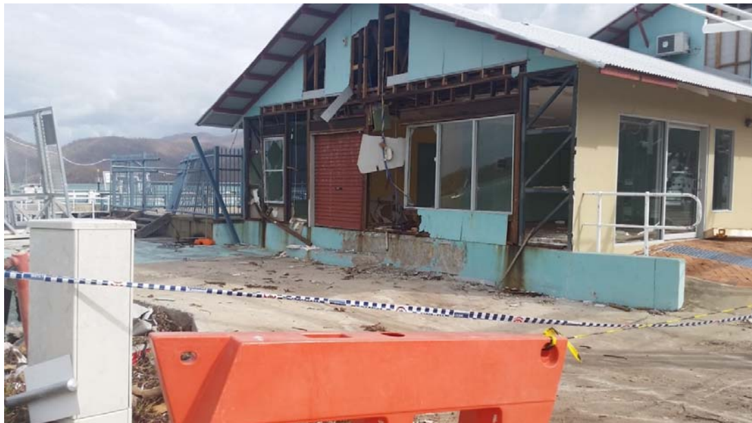
Figure 11. Extensive cyclone damage evident at Shute Harbour terminal
