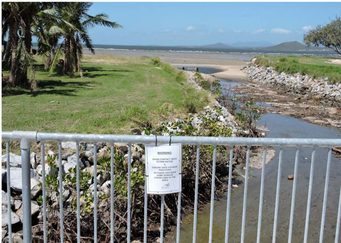
Figure 5. Sewage stormwater overflow into the ocean, Bowen
