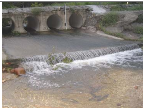
Fish migration barrier prior to construction – Fish accumulating downstream of water surface drop at culvert outlet apron (13/01/04)
