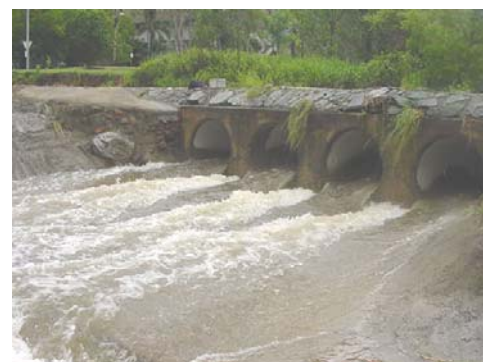
Fish migration barrier problems at pipe barrel and culvert outlet (-/02/02)
