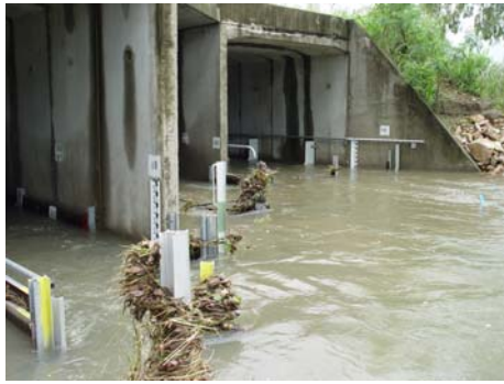
Inlet to culvert barrels with nib walls removed – Corner baffle fishway on right (02/02/07)
