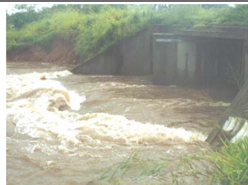
High velocity conditions and turbulent flow at culvert (-/04/00)
