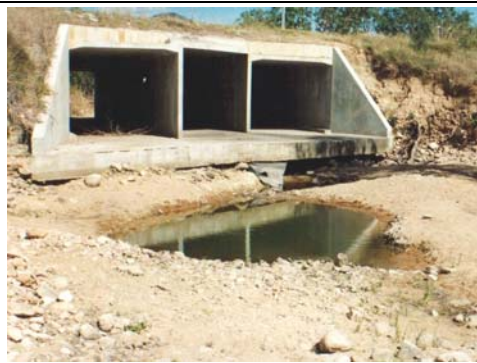
Box culvert in relatively steep gradient stream reach - erosion at outlet (-/06/97)
